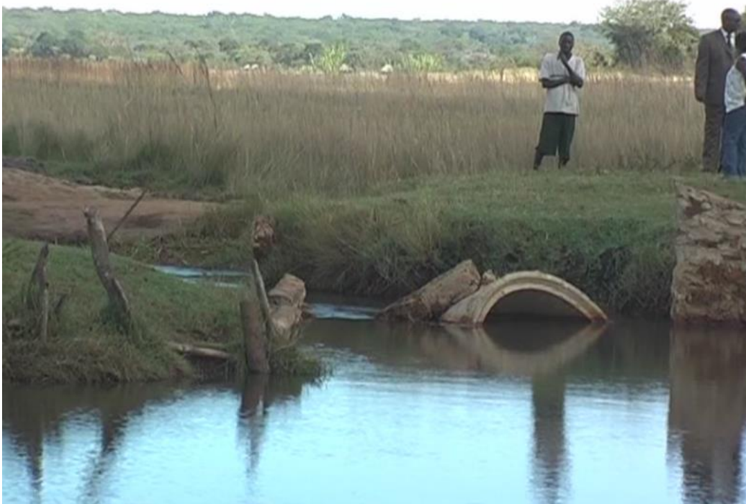
Poorly constructed culvert washed away
